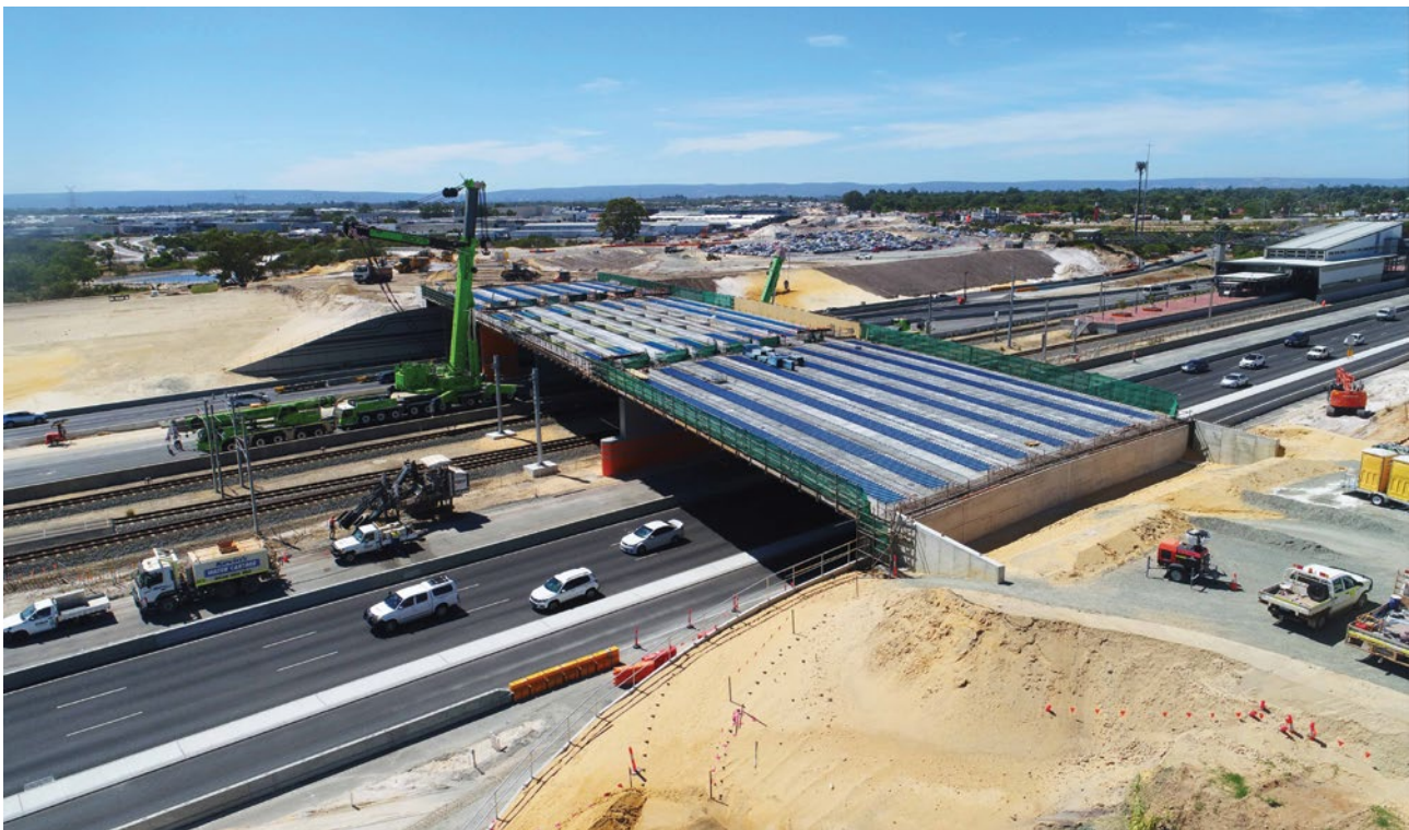
24 bridge beams installed over Kwinana Freeway, between Beeliar Drive and Berrigan Drive (Source: Main Roads Western Australia)
